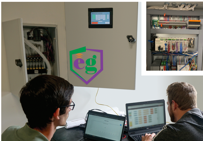
enVgrow engineers programming custom control panel
