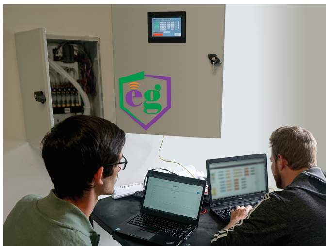
enVgrow engineers programming a custom control panel
